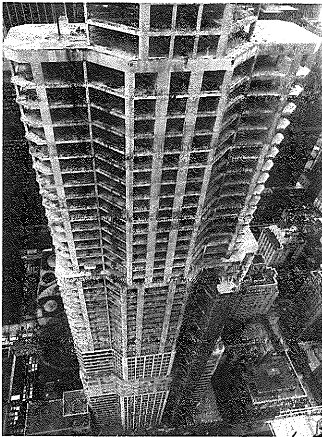
Fig. 10—City Spire, construction view, north elevation, showing setbacks and available Manhattan views (photo: Berenstein Associates)
